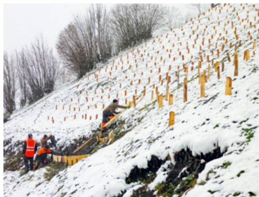
Figure 53 Stakes to protect an access road against gliding snow; the stake driving ratio of 2:1 in/above ground is essential.
