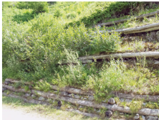
Figure 69 (left) and Figure 70 (right) Cribwalls stabilise vegetated slopes and merge into the landscape.
