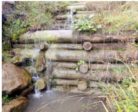
Figure 7 24-year-old wooden torrent dam (Hergiswil, Nidwald) with incipient wood decay in the area of alternating humidity on the right below the silted up section and the wing wall.
