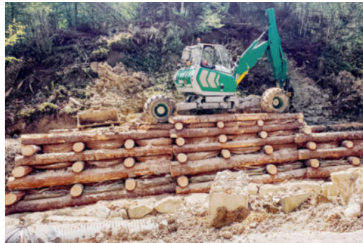
Figure 73 (left) Wooden crib to protect an embankment against erosion, using wood wool and willow cuttings.
