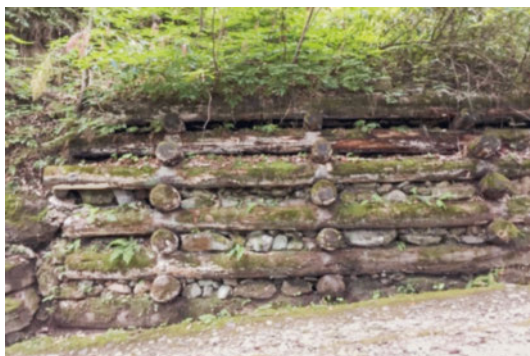
Figure 27 Example of an approximately 30-year-old wooden crib with stone infill, used to stabilise a road embankment.
