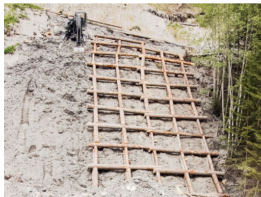
Photo in 2011 (left) Construction of slope grating with log diameters of 15 cm and a distance between the logs of 2 × 2 m.
