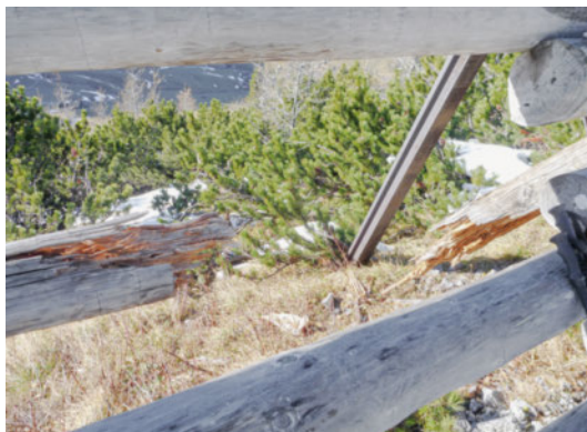
Figure 60 Broken rotten grate beam of a timber-steel snow bridge.
