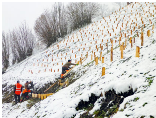
Figure 53 Stakes to protect an access road against gliding snow; the stake driving ratio of 2:1 in/above ground is essential.
