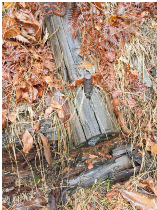
Figure 23 (left) Connection between transverse and longitudinal logs by means of a reinforcing bar.
