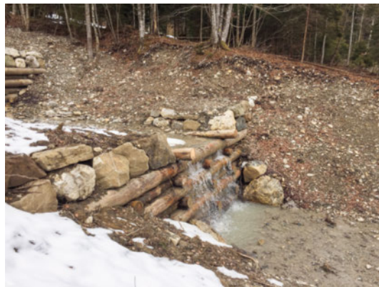
Figure 38 Left: Log crib check dam with wing walls made of armourstones and roundwood log infill. Right: Toe scour zone protection constructed from armourstones.
